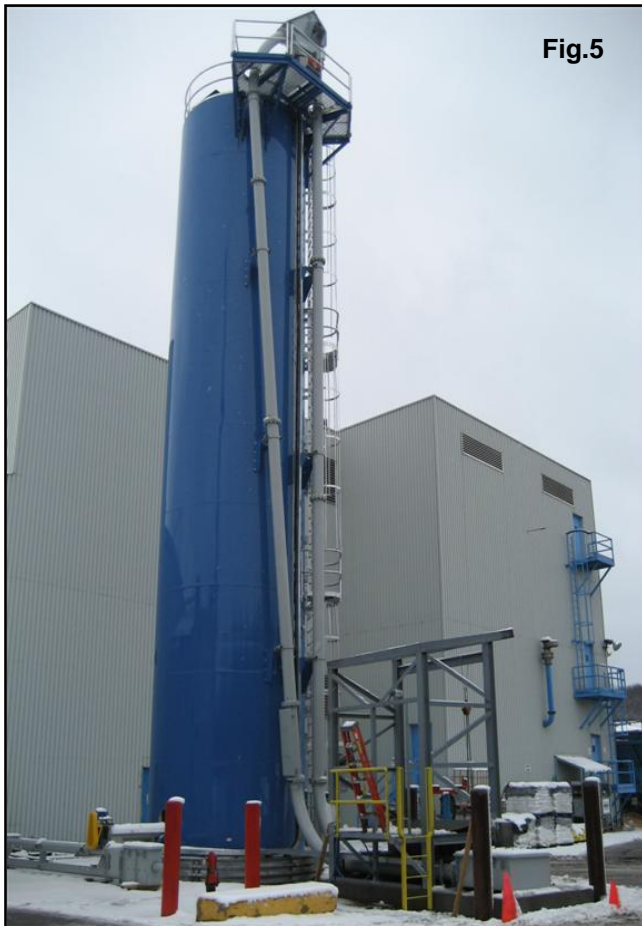
Truck Discharge to a Silo
