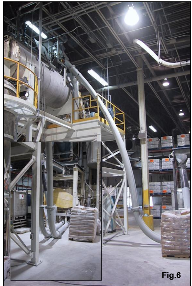
Blender, Manual Dump Station Feed to a Wet Mixer in a height restricted area.
